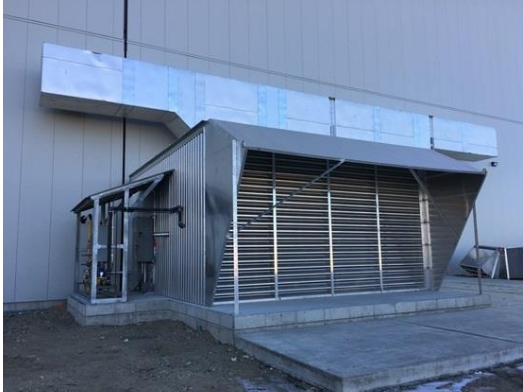
Conventional Outdoor Air Make-up Unit
